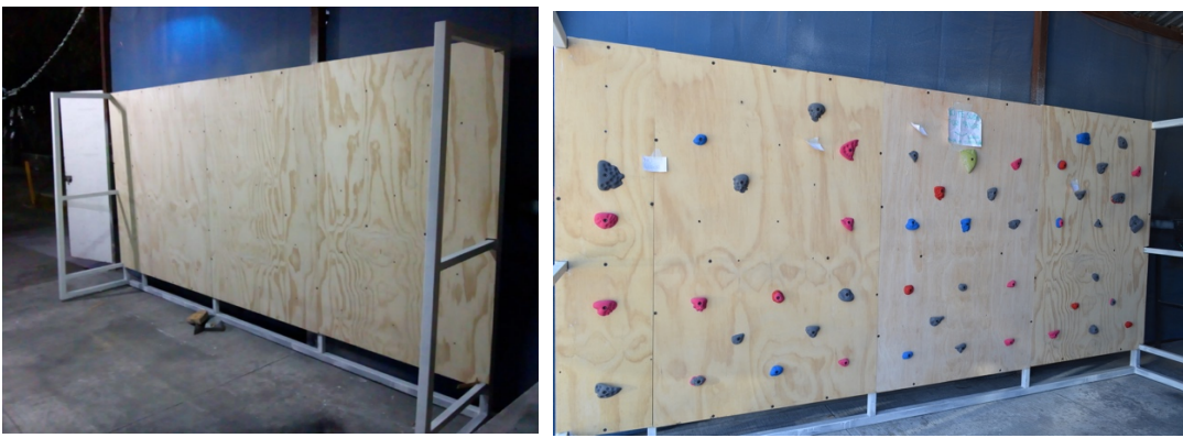
Figure 4: Construction step by step of the climbing wall prototype. Source: Own Elaboration
